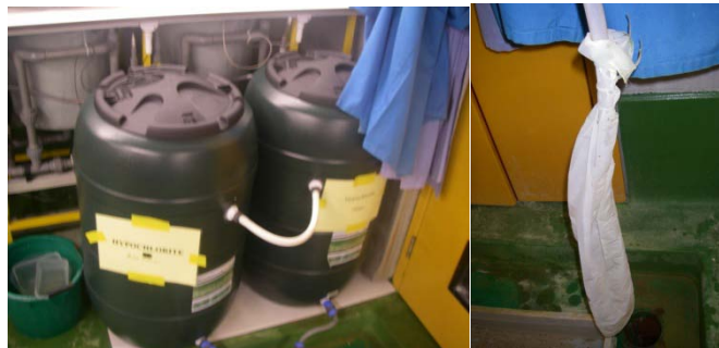
Figure 2- Water butts used for disinfection of waste water and fine mesh sock on outflow.
