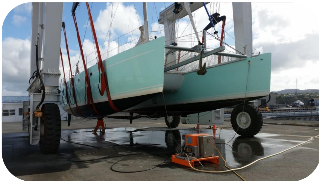
Example installed washing station
